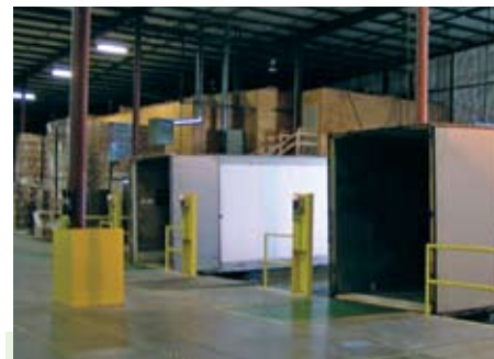
The open interior dock area before Zoneworks wall were installed. Large overhead dock doors allowed cold air into the facility making employees uncomfortable and increasing energy costs to heat this area.
